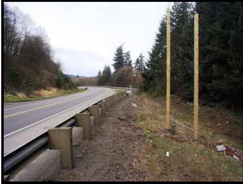
Photo 5: BEFORE – Shows the work zone site during 1st post-incident FACE investigation site visit, prior to fill, rock and gravel being brought in to augment the sign installation. Looking west along the eastbound lane of highway.
