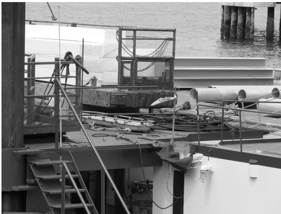
Photo 4: Upper deck of barge where victim was welding a broken railing (photo taken shortly after incident).
