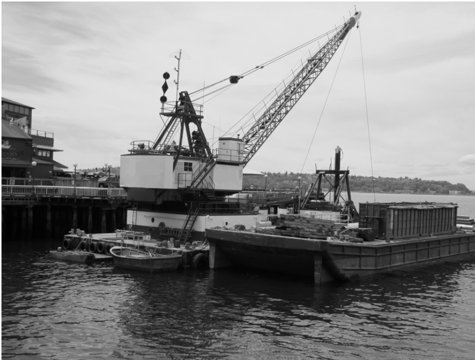
Photo 2: Crane barge and barge used for construction supply storage and waste materials at incident site (photo taken shortly after incident).
