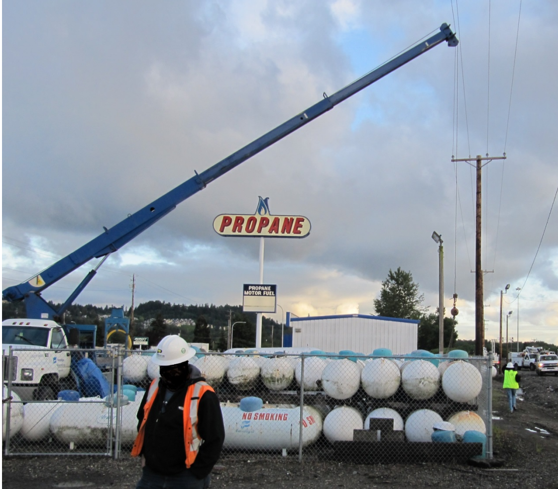
Photo 10. Crane boom tip contacting eastern phase wire of a three-phase 7,200 volt power line. The power lines were located to the west of the yard, and for a short distance inside the yard, and ran north and south. The sequence of the three-phase 7,200 volt power line wires in relationship to the crane boom is eastern phase, neutral, middle phase, and western phase.
