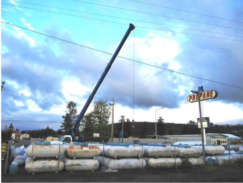
Photo 4. Incident site showing the employer's propane tank storage yard with 320-gallon capacity propane bulk storage tanks that the victims were inventorying. The photo was taken after the crane boom made contact with the energized 7,200 volt power line.
