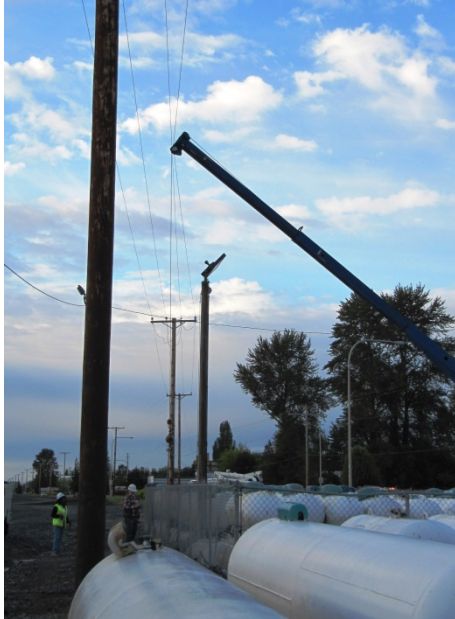
Photo 9. Incident scene with crane boom contacting power line.
