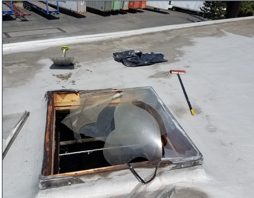
Skylight through which the roofer fell 30 feet.
