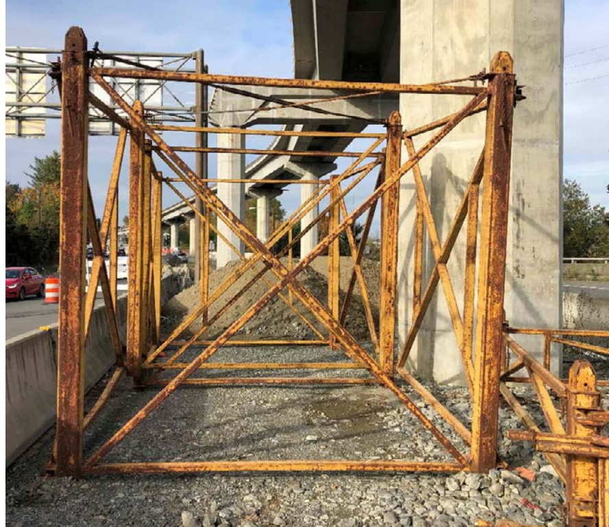
Photo 3. Incident scene shore tower section.
