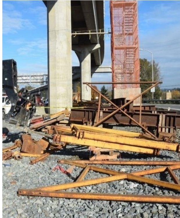
Photo 1. Incident scene beneath an elevated section of a light rail line under construction.
