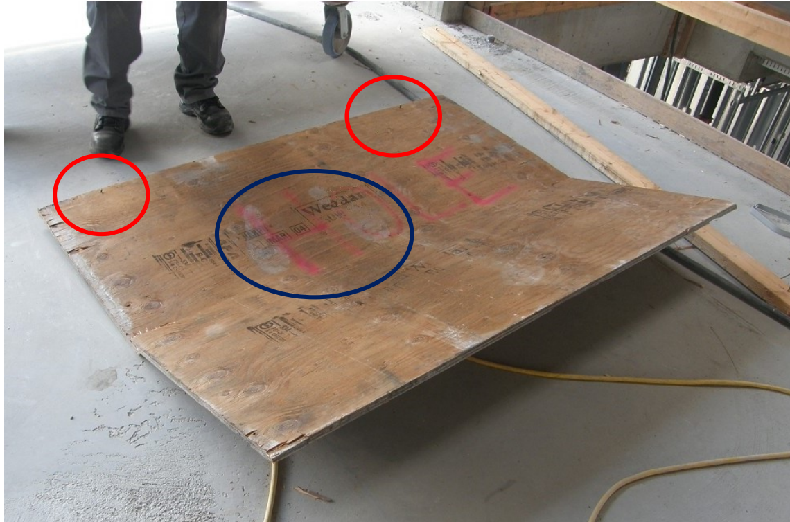
Photo 5. Plywood hole cover that failed with the word “HOLE” painted on it. Two nails that secured the cover to the stub wall sill are indicated by red circles. The ironworker’s boot prints are indicated by the blue circle.
