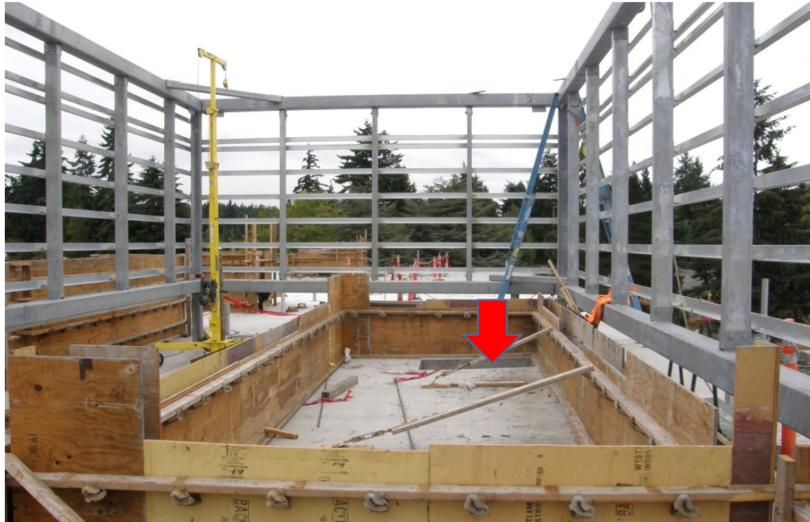
Photo 2. Incident scene showing rooftop windwall structure, wooden form for a concrete stem wall to support an HVAC unit, and the location where the ironworker jumped down from the form onto the hole cover.
