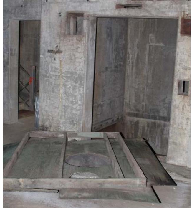
Elevator shaft where grip fell with wooden guard on the floor that used to cover shaft opening.
