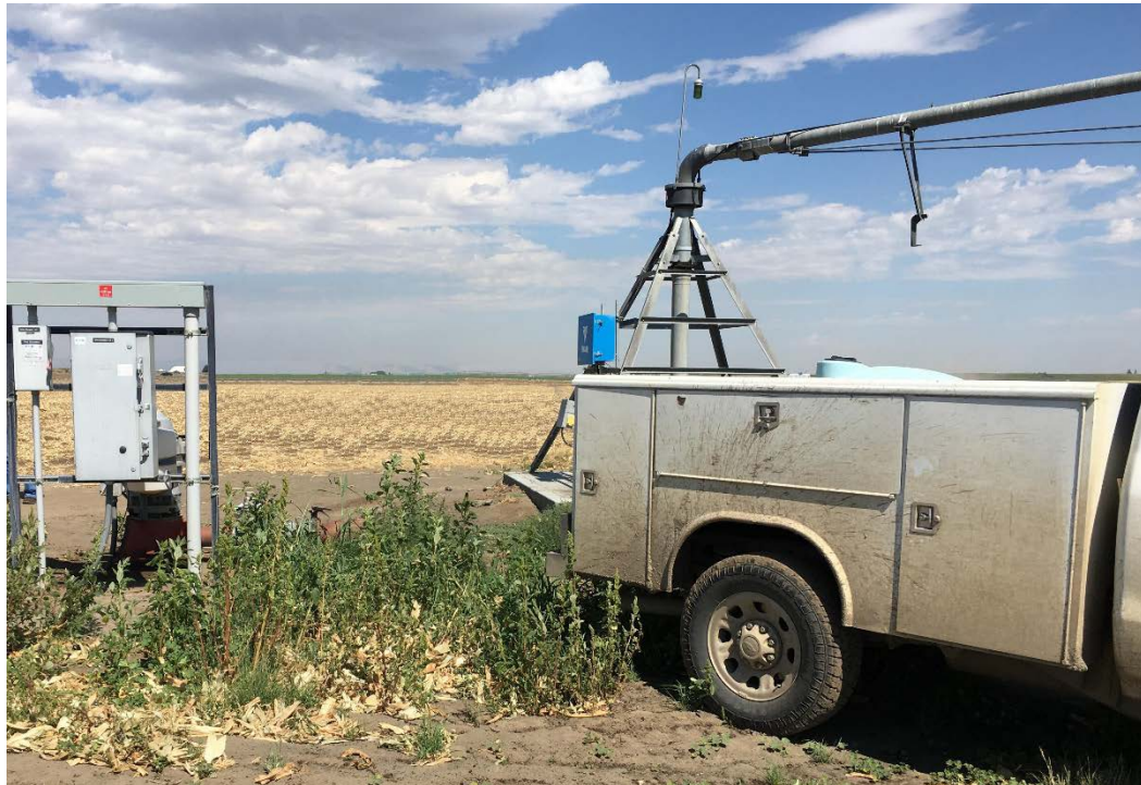
Photo 3. Vegetation blocking operator's view of water main.
