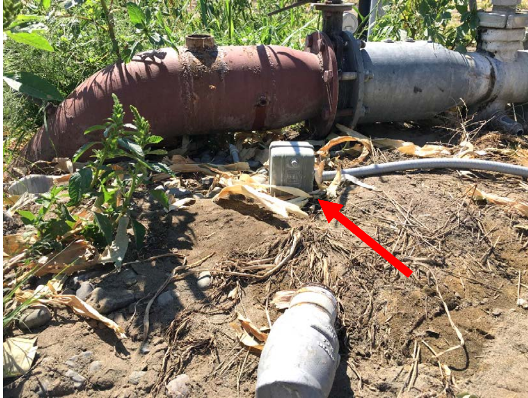
Photo 2. Pivot water main with broken water flow regulator and pressure switch (indicated by arrow).
