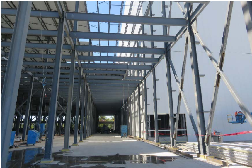
Photo 2. Interior view of incident scene at the cold storage facility under construction.
