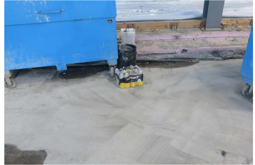
Photo 3. Area where the apprentice ironworker went to retrieve a bottle of water when he was struck by the dropped steel wedge.
