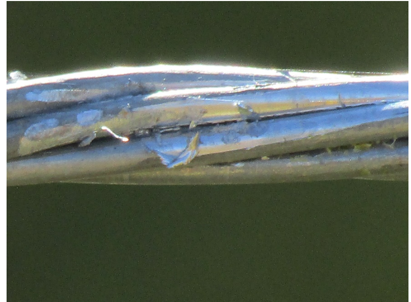
Photo 4. Cross-cable with abrasion where it may have snagged on hex-head bolt.
