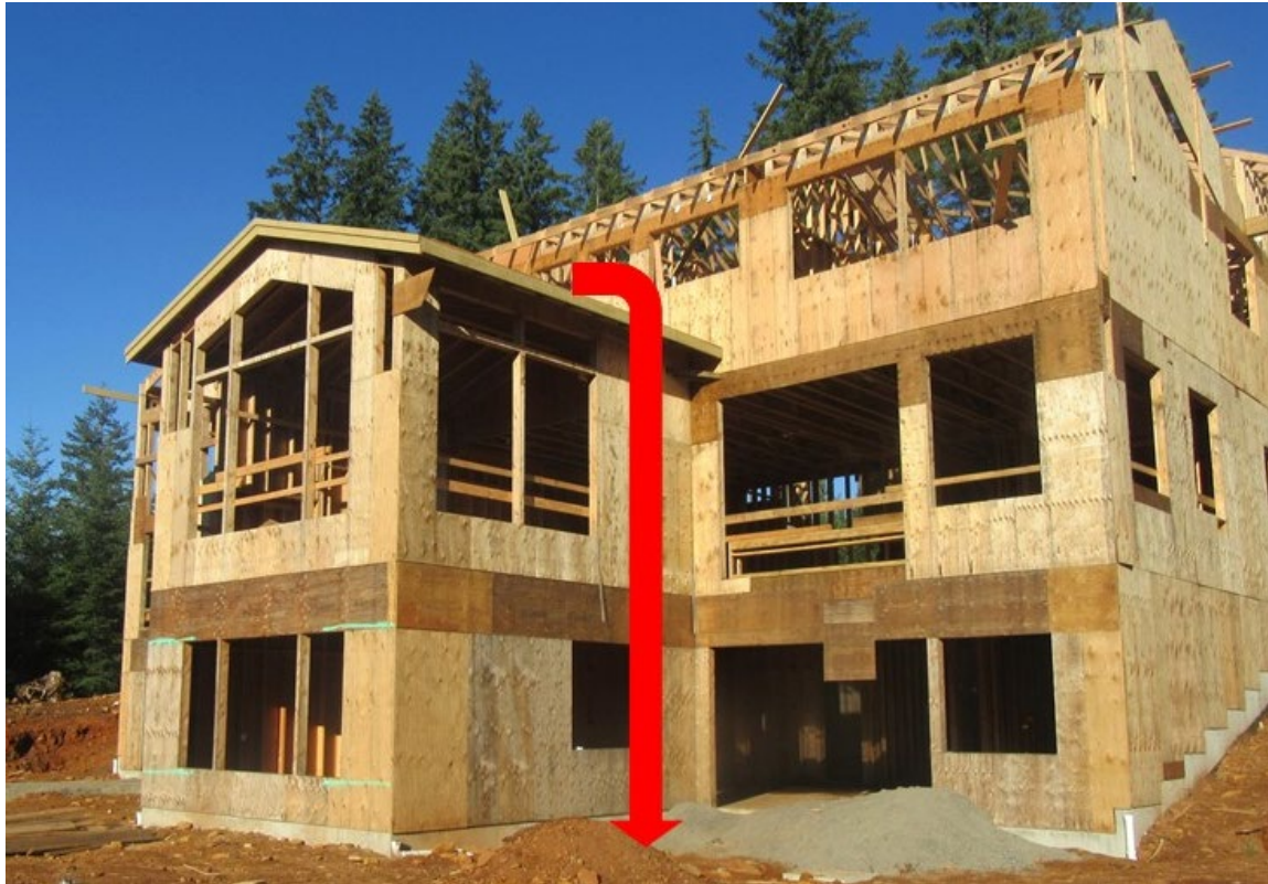
Photo 1. House where framer fell 25 feet from the lower back sheathed roof. He was not using fall protection
