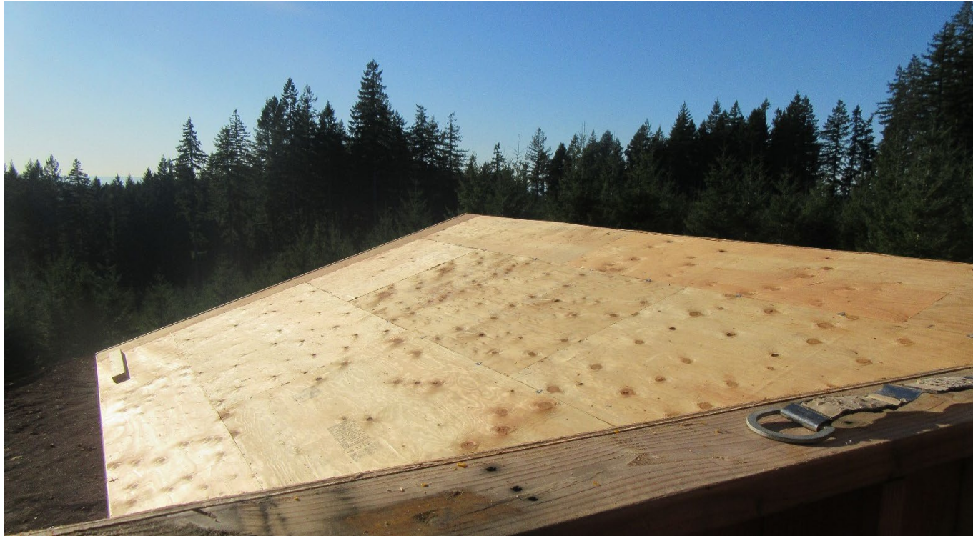
Photo 3. View from above the sheathed lower backside roof. The framer fell from approximately halfway along the left side edge. An anchor point on the window sill is visible in the lower right.
