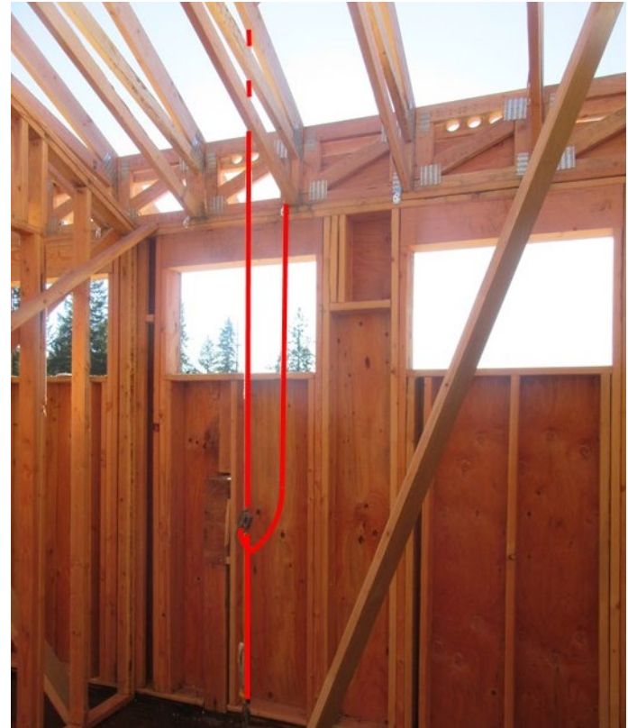
Photo 5. Lifeline that could have been used. The roof the framer went onto is on the other side of the wall.
