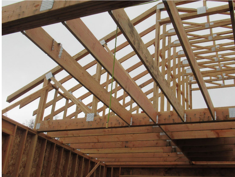
Photo 2. View of the second story floor joists from inside the garage. The shaded area in the floor joists on the right side of the photo is the pile of OSB sheathing they were using to lay the floor.
