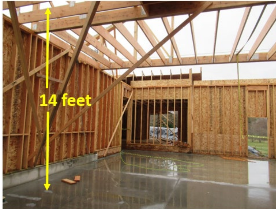
Photo 4. View of the inside of the garage in the area the carpenter fell. The distance from the top of the floor joists to the concrete floor measured 14 feet.
