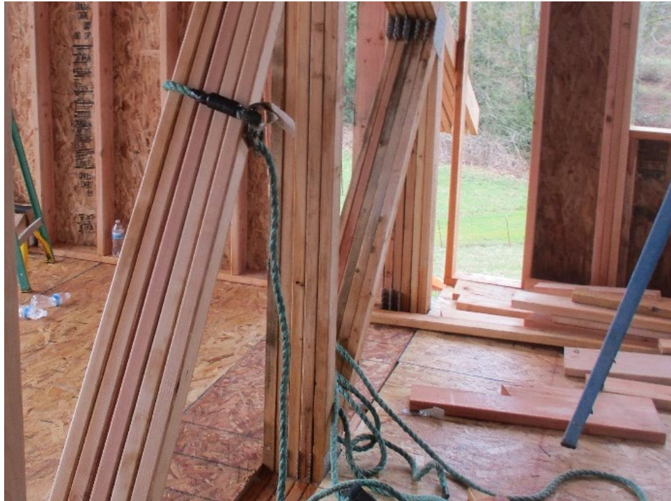
Photo 5. Demonstration of how the crew wrapped their fall protection system life line and looped it into itself around a diagonal set of 2x4s installed as one of the truss cross-braces.
