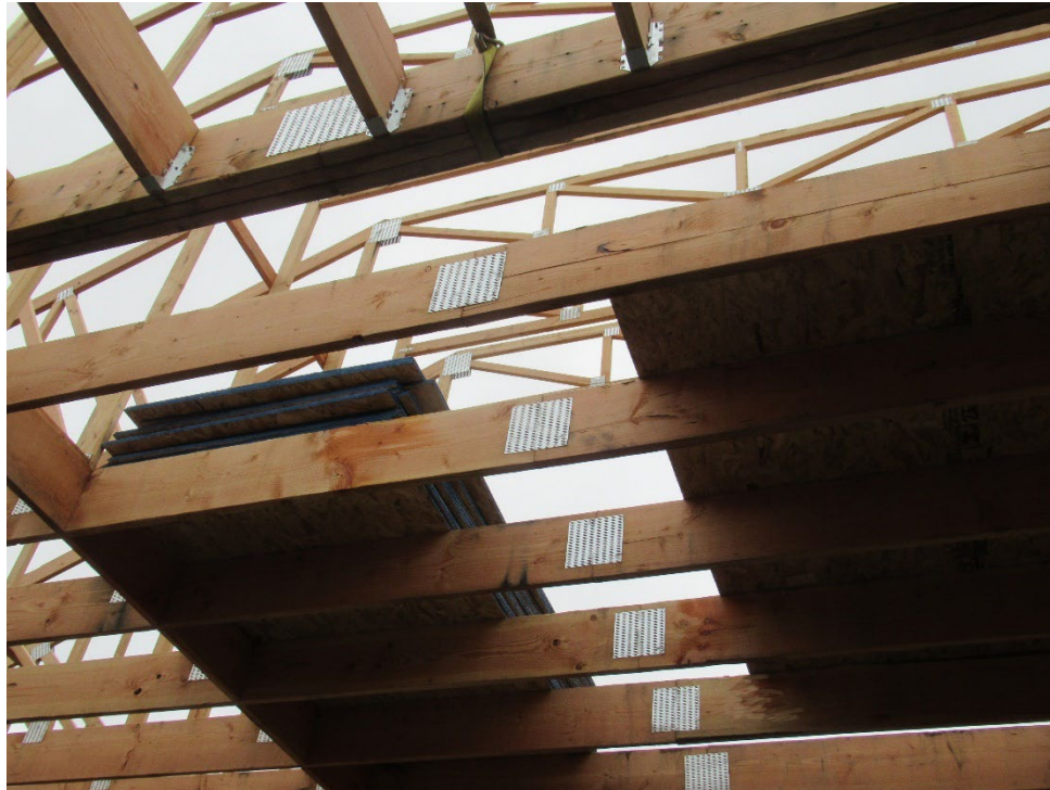
Photo 3. View of the floor leading edge and the pile of OSB sheathing they were using to lay the floor.
