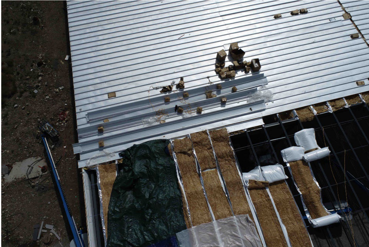
Photo 2. View of the area where the roofers were working and the leading edge they were constructing near where the roofer fell.
