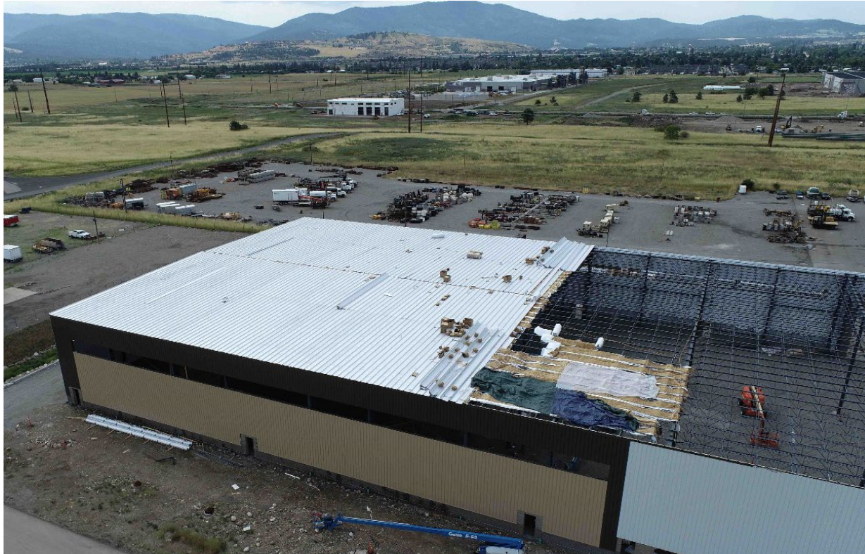
Photo 1. View of the incident scene where the roofers were installing the low-pitch metal roof. The mobile elevating work platform used to access the roof is in the bottom center of the photo.
