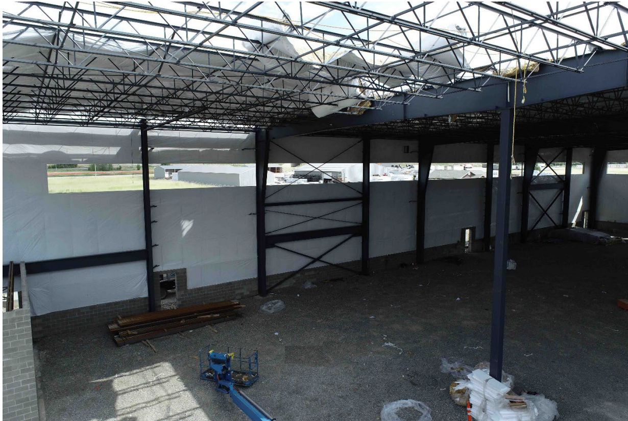
Photo 4. Inside of the warehouse where the roofer fell onto the gravel floor while constructing the leading edge of the roof.
