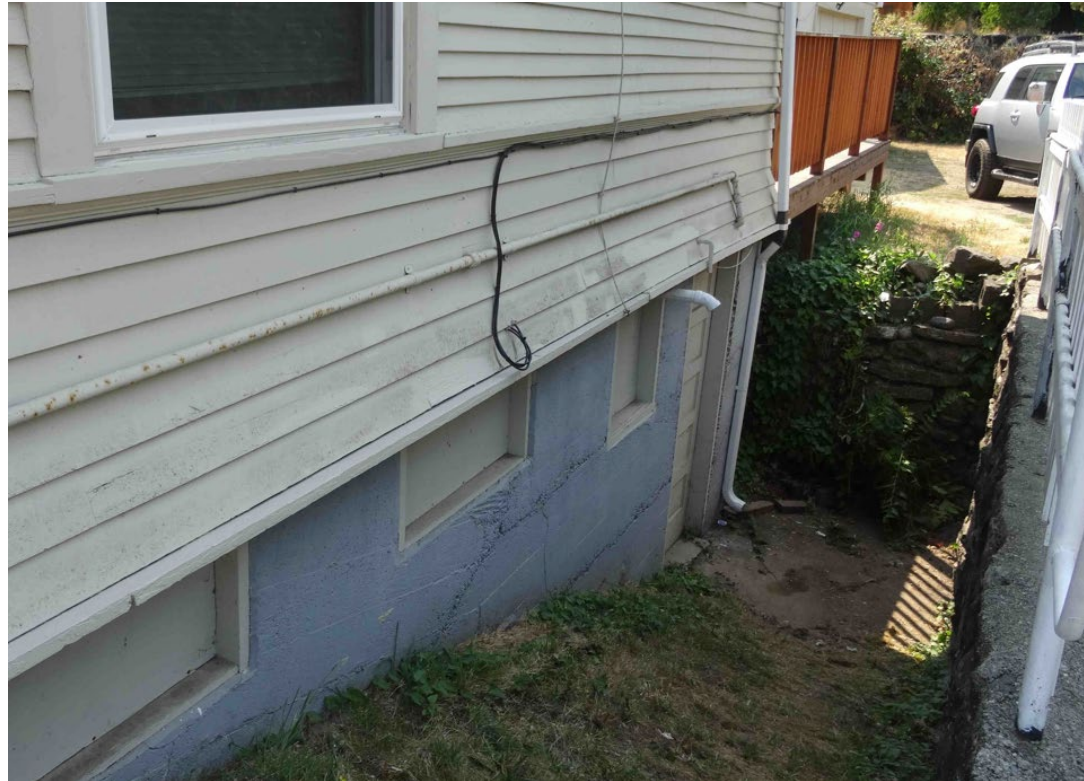
Photo 2: Below-grade 6-foot rock retaining wall and basement entrance. The ladder appeared to be used for climbing between the two levels of ground.
