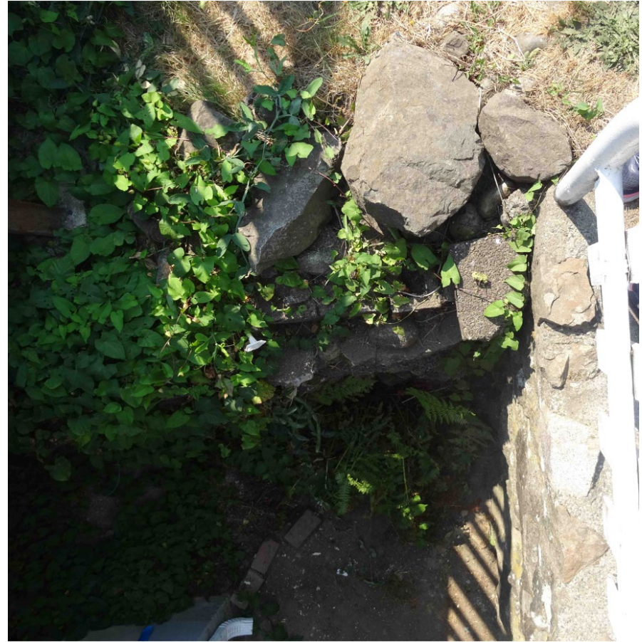
Photo 4: Loose rocks at top of retaining wall.
