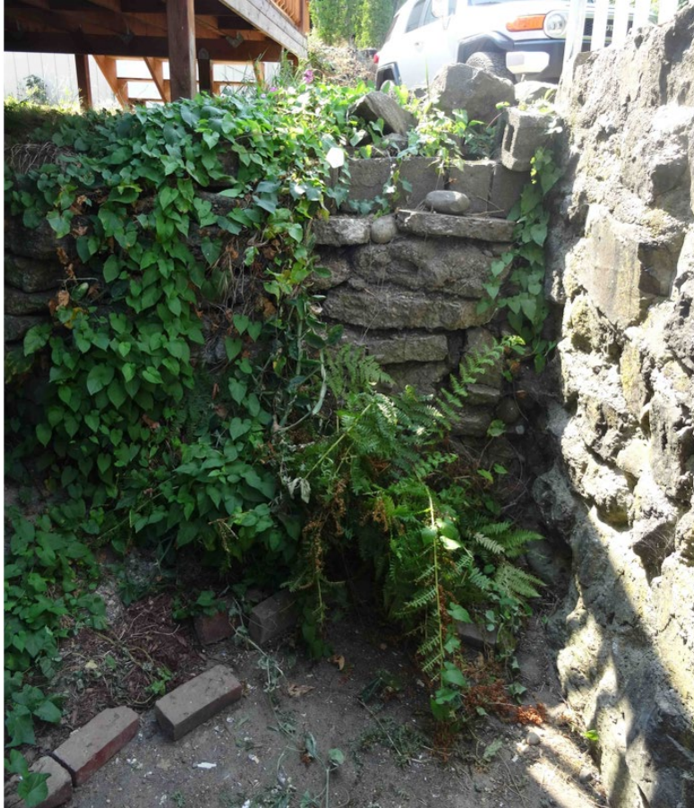
Photo 3: Rock retaining wall the ladder was leaning on.
