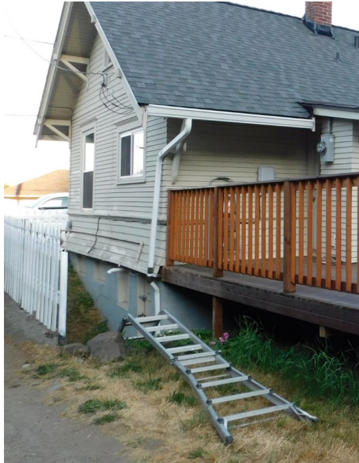
Photo 5: Unsecured top half of ladder folded over the retaining wall and resting on the grass surface.
