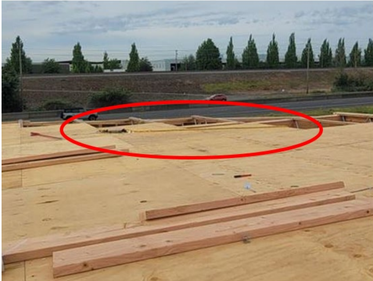
Photo 3. Fall protection anchor, shock-absorbing lanyard, and lifeline near roof deck leading edge where worker fell.
