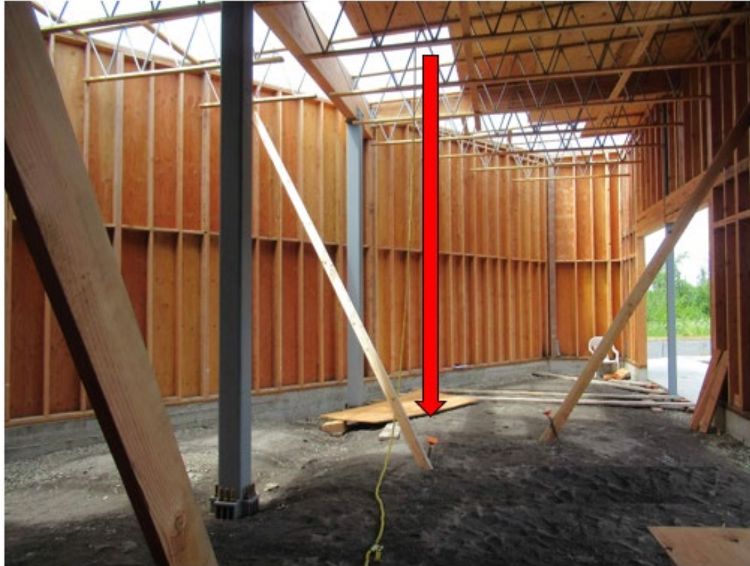
Photo 2. Wider view of building interior where worker landed after falling from leading edge of roof deck above. Arrow shows direction of fall.
