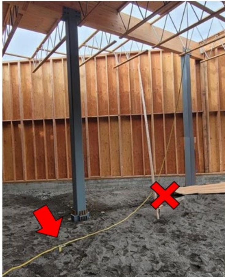
Photo 1. Lifeline with rope grab stretched to show length from where worker fell (X) near plywood sheet.
