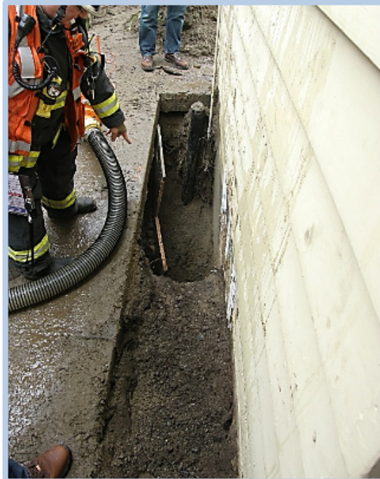
The collapsed trench after the victim's body was recovered.
