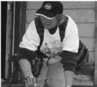
Mary Dunn, a fourth year apprenticeship student and employee of Biwell Construction works to restore a deck during Rebuilding Together Seattle 2006.
