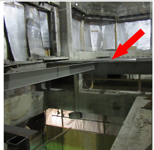
Area where workers were setting a steel beam over an old elevator shaft. The ironworker was sitting on the edge of the metal deck to secure the beam (arrow).
