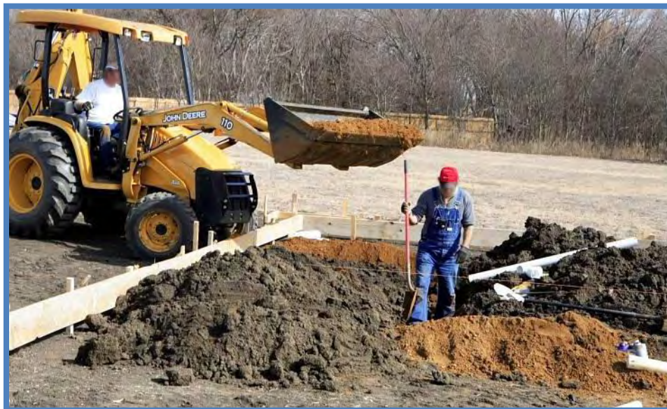
Trench digging: Workers should not stand near or under operating machinery. Spotters should be used if machine operators cannot see workers inside a trench area. Image courtesy of OSHA Training Institute, Southwest Education Center / elcoshimages.org.
