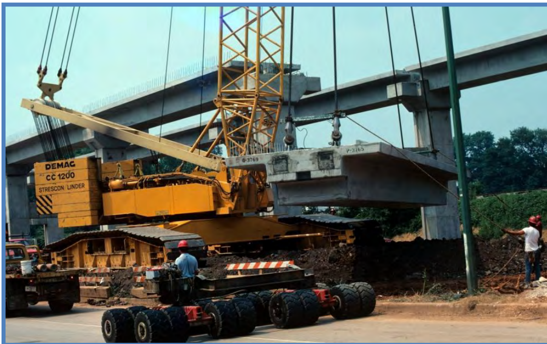
Crane lifting bridge section: Workers should never work, stand, or place themselves below suspended loads. Image courtesy of NIOSH/John Rekus/elcoshimages.org.
