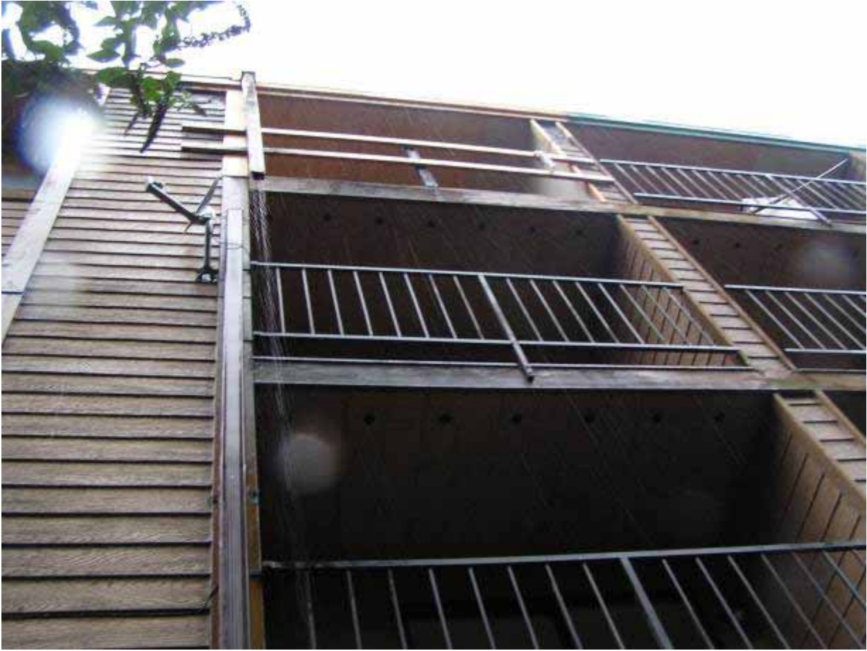
Figure. The apartment balcony with a temporary guardrail re-constructed after the incident.
