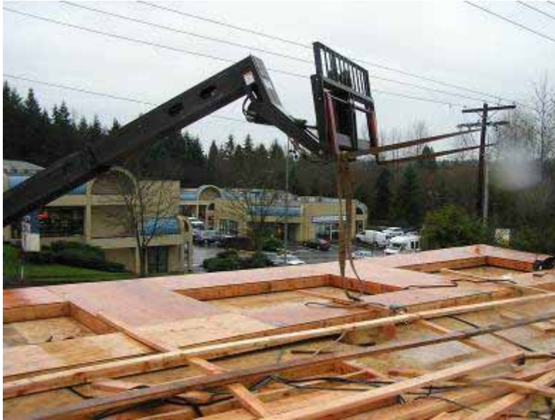
Photo: This picture shows the fallen wall and the forklift with the attached nylon strap after the incident.
