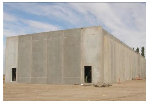
The precast concrete building where the victim fell through a skylight roof opening.
