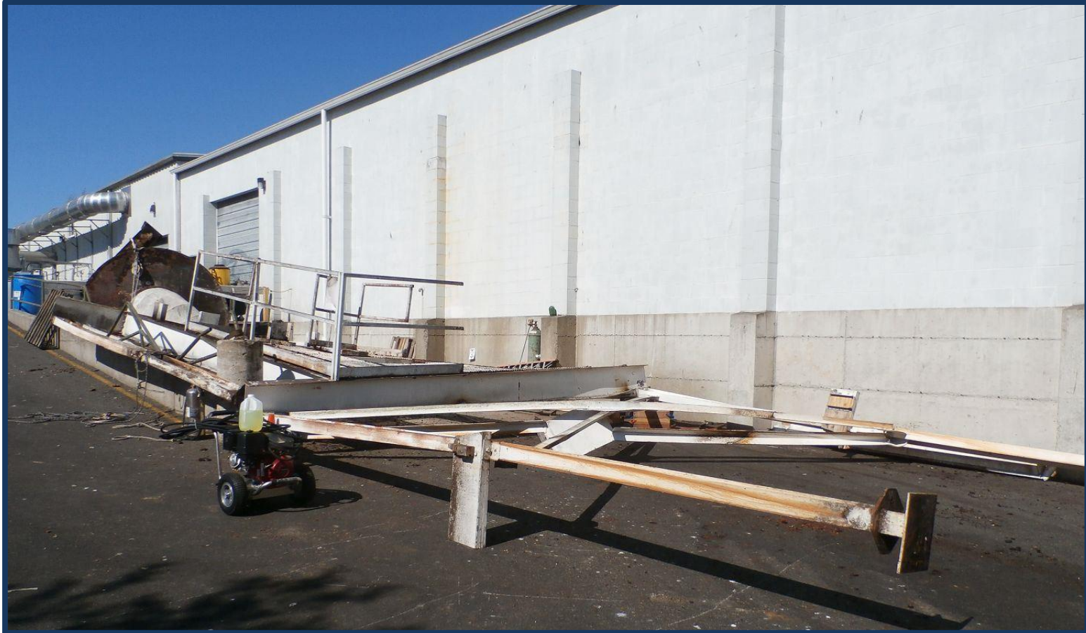
Incident scene showing the collapsed steel supporting structure for a cyclone air separator.
