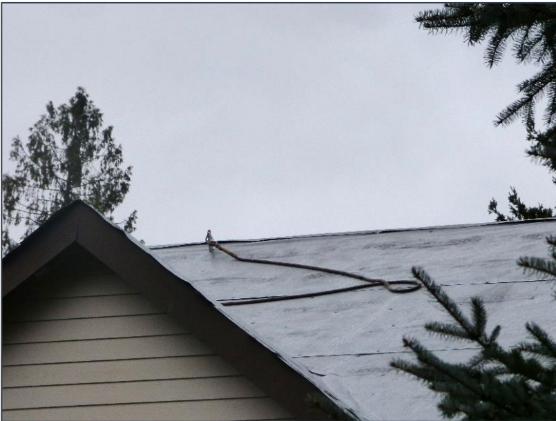
Photo 2. Roof of the house showing the location of the lifeline for rope grab attachment.
