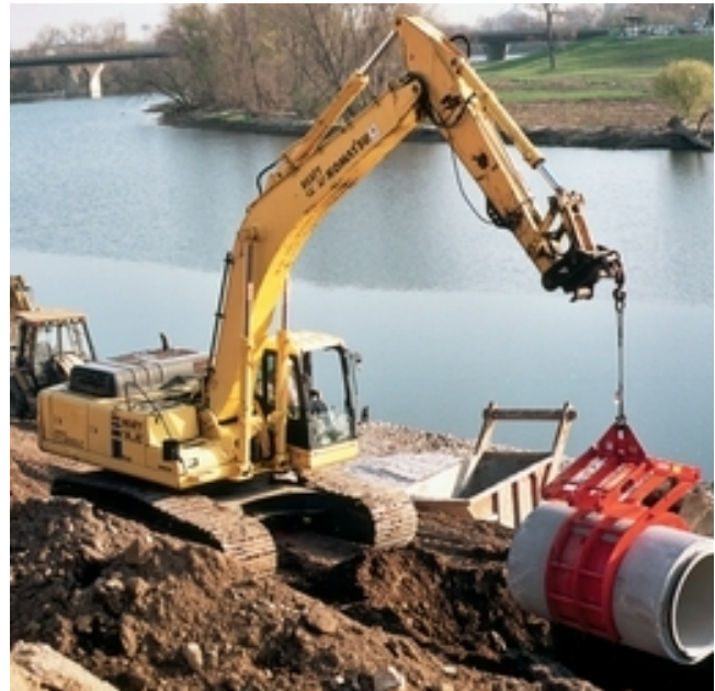
Photo 2: Photo of an excavator completing an over the front lift. Notice the cab and counterweight are in line with the tracks
