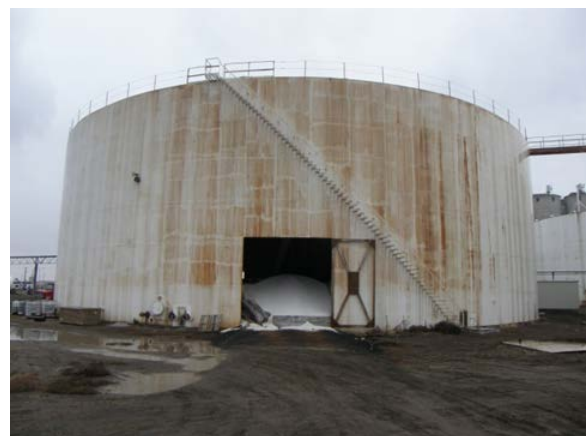
Photo 2: Steel tank used for bulk fertilizer storage
