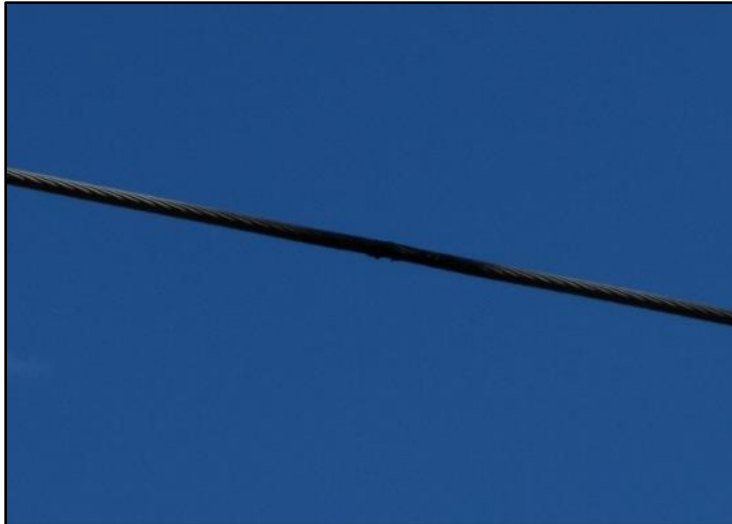
Photo 3: Burn damage on power line where tree fell onto it
