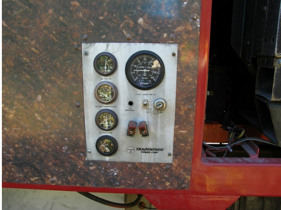
Photo 13: Engine controls for the blower system. The engine's power is controlled by using a key.
