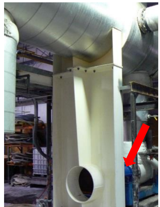
Photo 2 Recirculation pump location behind heat exchanger support column.
