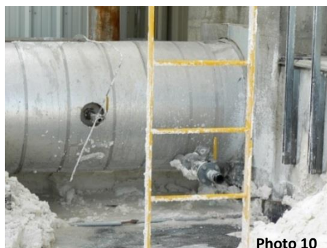
Photo 9 Boric acid evaporation system drain valve at time of incident.
