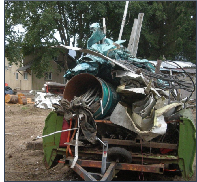
Photo 4. Incident site with trailer loaded with scrap.
