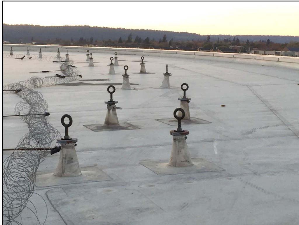
Library building rooftop anchor points. The victim did not use any of these.
