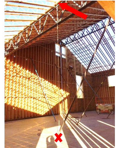
Location where the laborer fell from the roof deck (arrow), and where he landed on the floor ("X").
