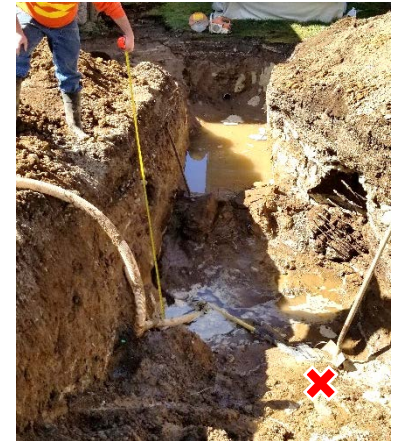
Unprotected trench after its sidewall collapsed. The “x” indicates the laborer’s location.
