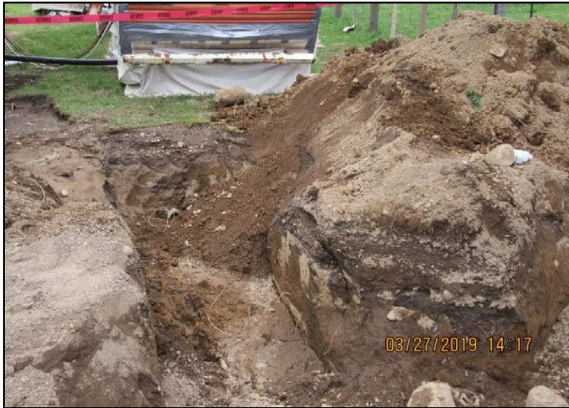
Photo 4. Spoils piles sloughing into the trench.
