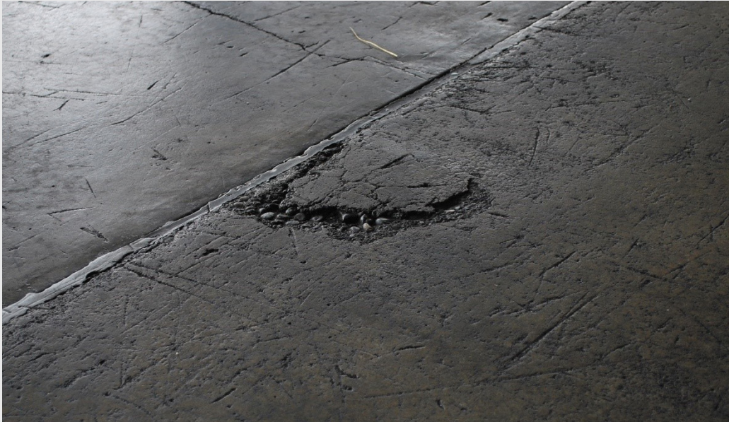
Worn pavement and work floors are common terminal yard trip hazards.
