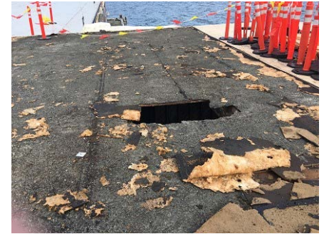
Rotten roof that the roofer fell through.
