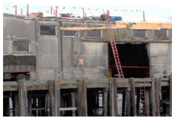
Area of building where the roofer fell through rotten roof.
