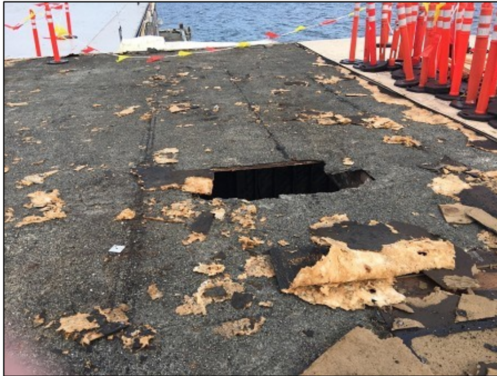
Photo 1. The rotten patch of roof that gave way when the roofer stepped on it.
