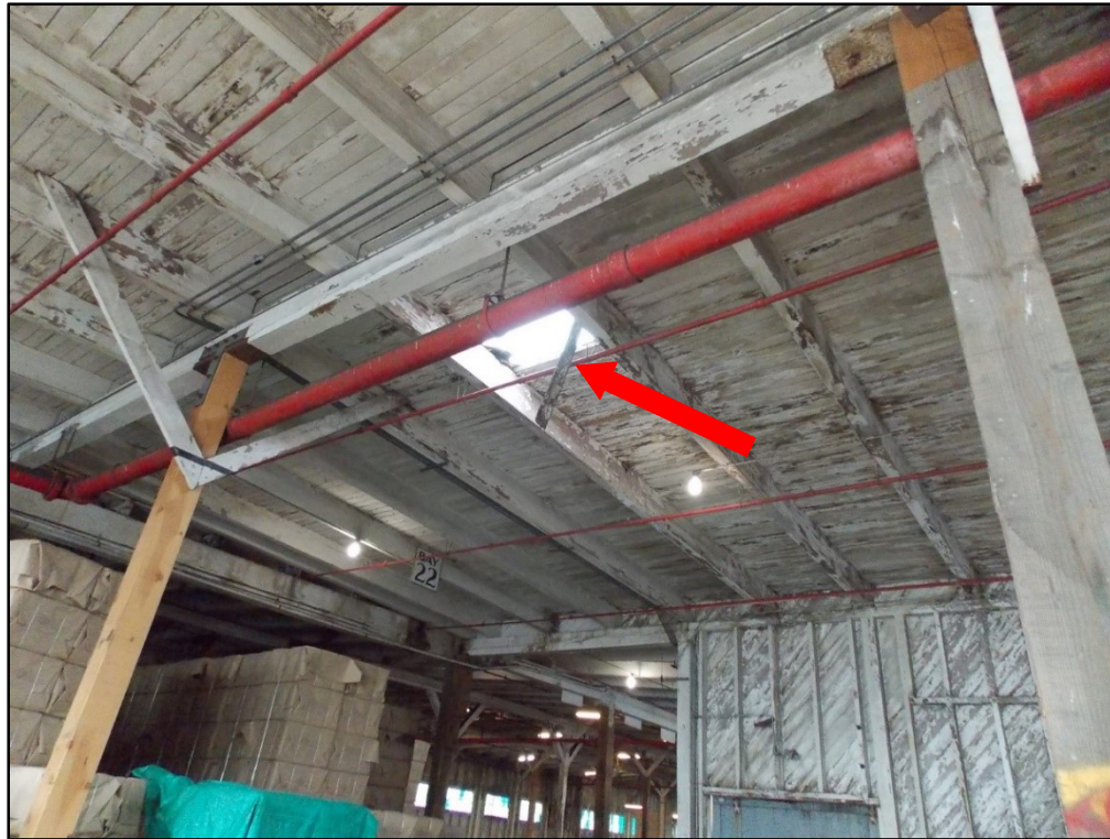
Photo 2. Hole created when the roofer fell through the roof. He landed on the floor 20 feet below.
