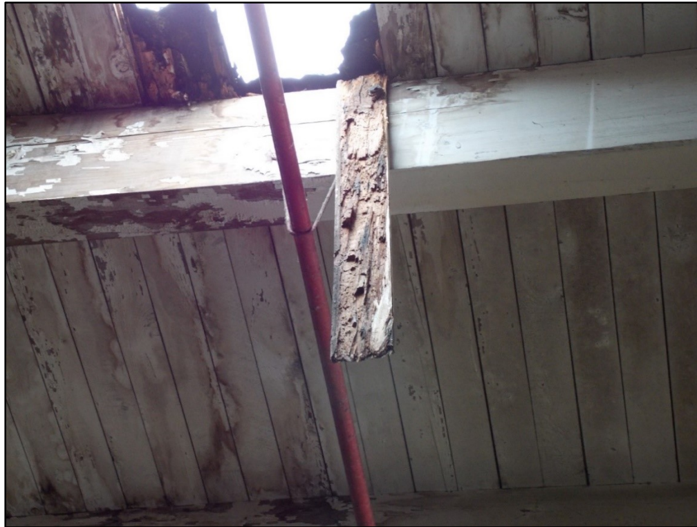
Photo 3. Close up of the roof hole that the roofer fell through showing the rotten wood.
