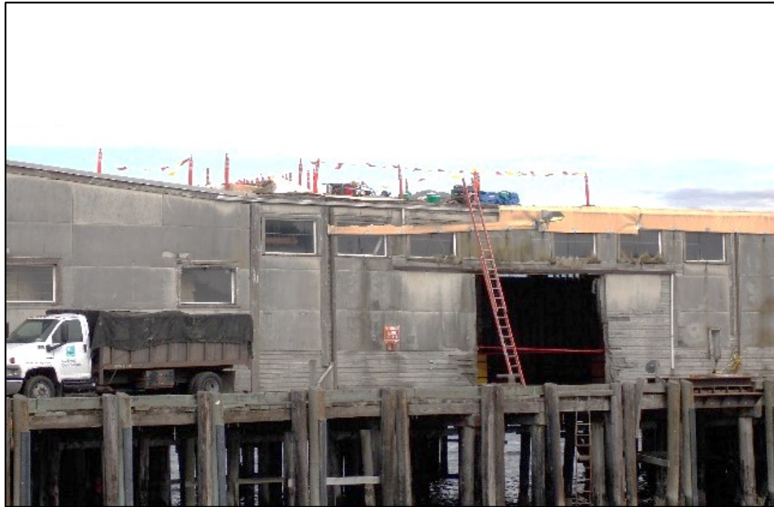
Photo 4. Building area where the roofer fell through the roof.
