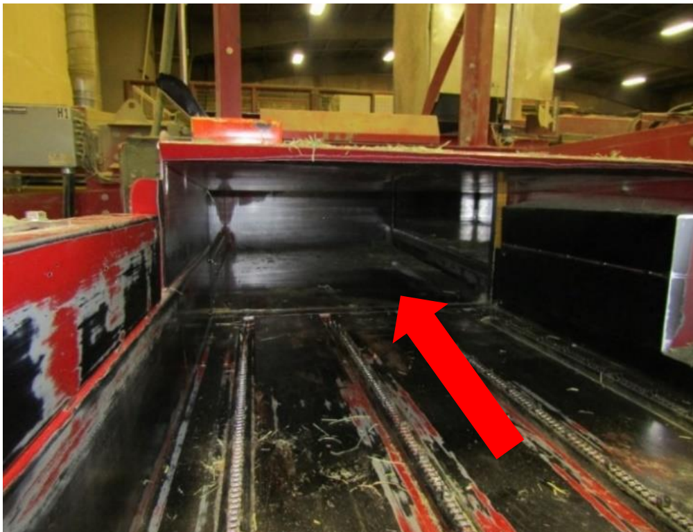
Photo 9: The red arrow shows where the operator crawled onto the scale pan that triggered the guillotine to raise up and nearly decapitate him.
