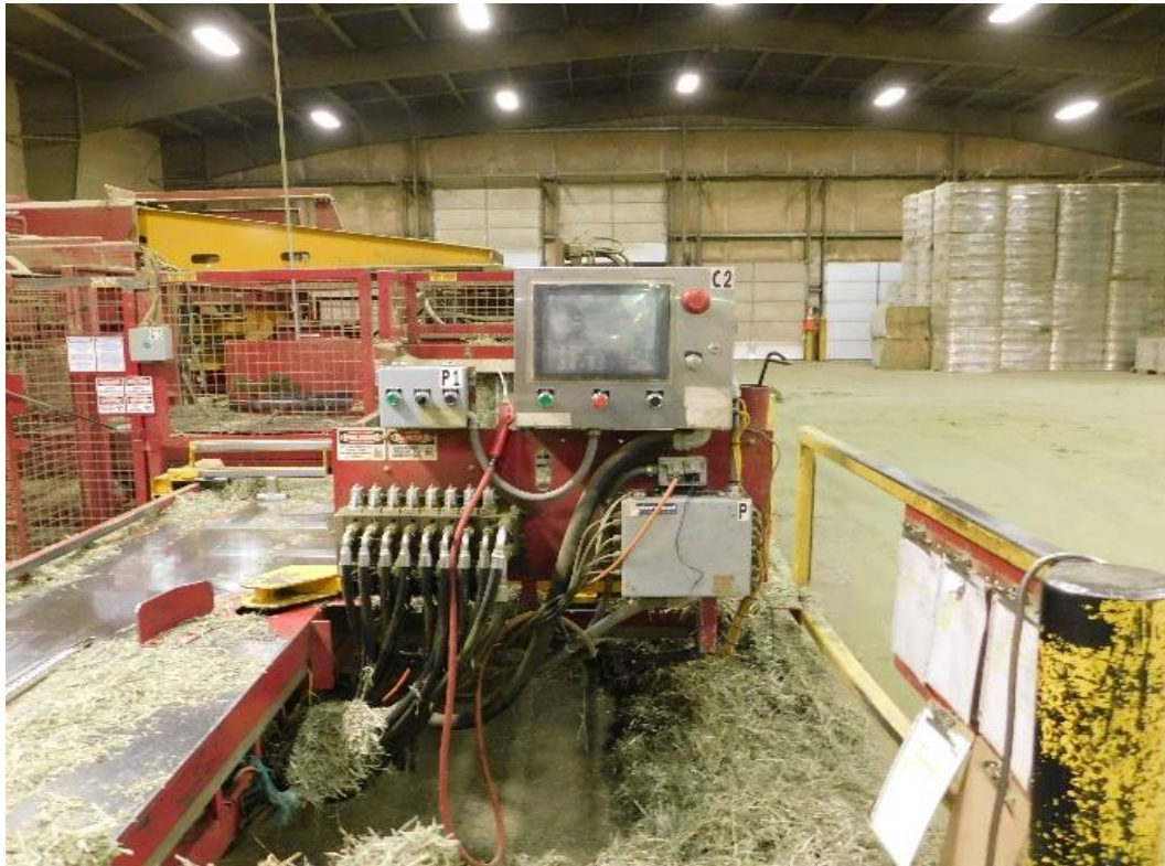
Photo 6: Operator's station with touchscreen interface panel.
