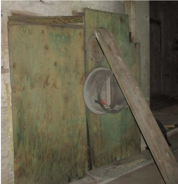
Photo 8: Elevator shaft guard as originally installed with round opening to allow air to flow and pressure to balance between elevator shaft and the room and wood plank for support. The guard was not fastened to the wall around the shaft opening.
