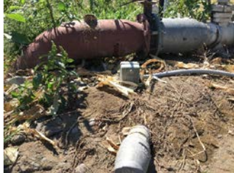
Pivot water main with broken pressure switch and water flow regulator.
