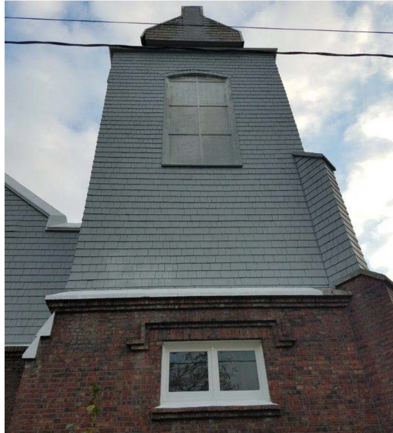
Photo 3. View of the church steeple and proximity of the overhead power line.
