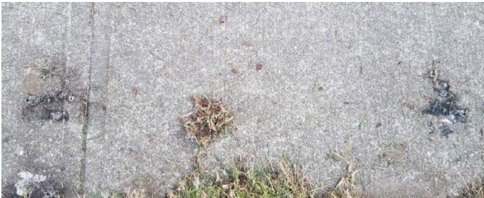
Photo 6. The sidewalk with burn marks where the ladder had been placed.
