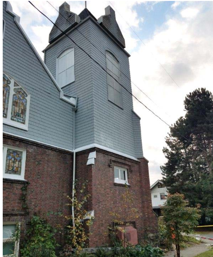
Photo 2. View of the church exterior where the extension ladder contacted the overhead power line.
