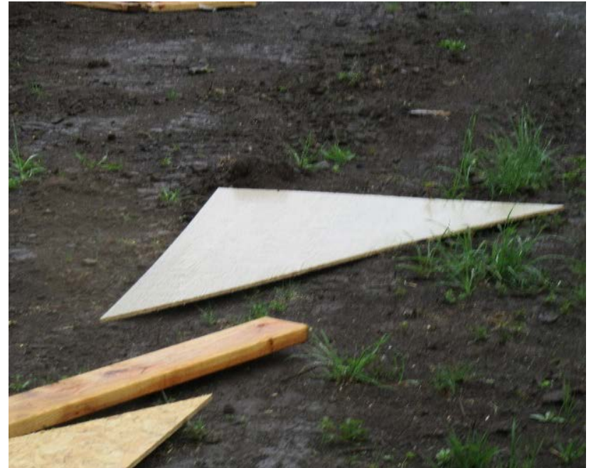
Photo 3. Plywood sheeting that framer was intending to place on the house gable.
