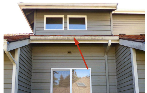
Figure 1: Red arrow shows the roof edge the foreman fell from while moving materials.
