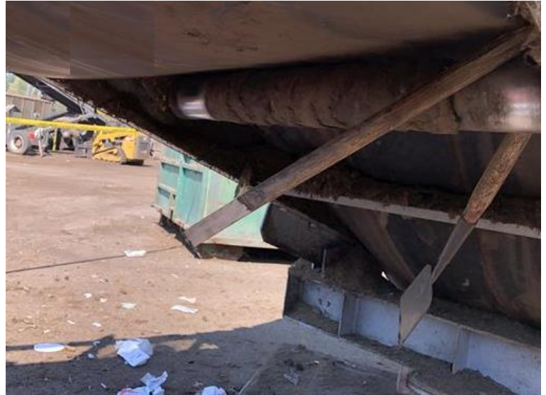
Conveyor belt and unguarded steel return idler roller with metal spade scraper tool that was pressed against the lead operator's throat. Responding workers cut the belt and broke the tool's wooden handle to release the operator. Photo taken after incident.
