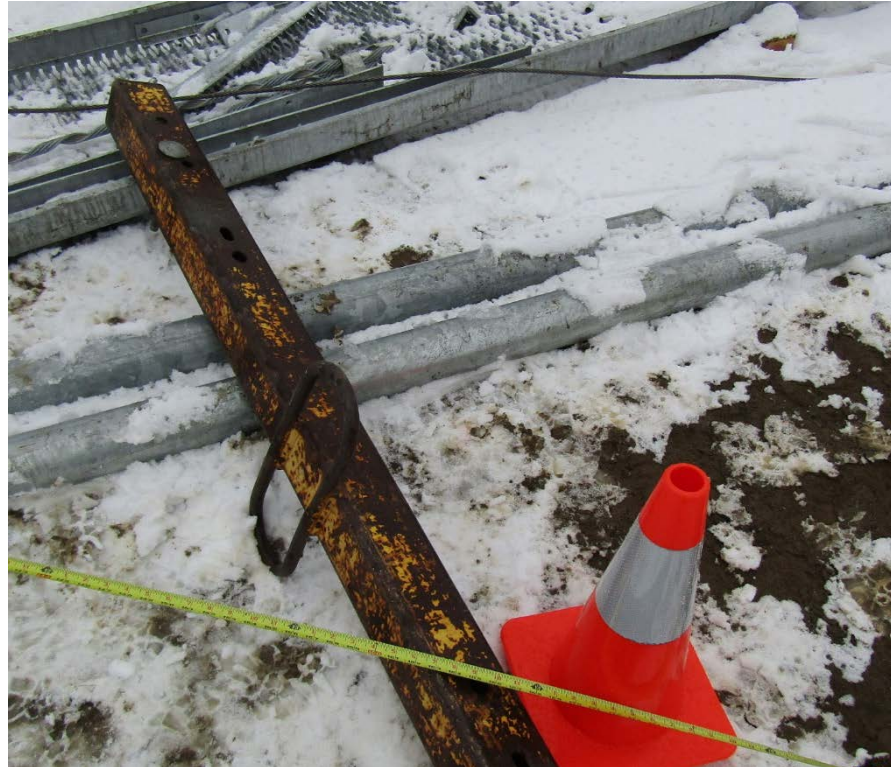
Photo 6. Steel jump plate used by the crew during tower erection with loop welded in the center.
