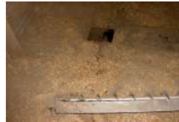
1: Keep safety covers on floor auger openings and use appropriate safety guards on sweep augers ( WAC 296-307-29005 ).
