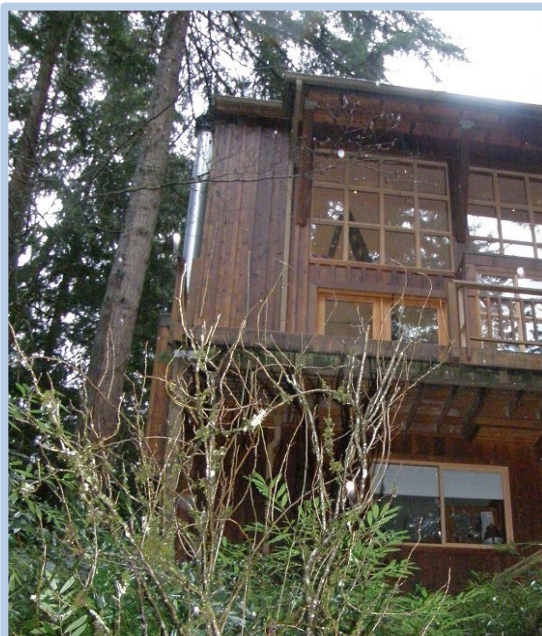
Photo of incident scene where a roofing contractor fell 35 feet from a roof and his employee fell from a ladder.
