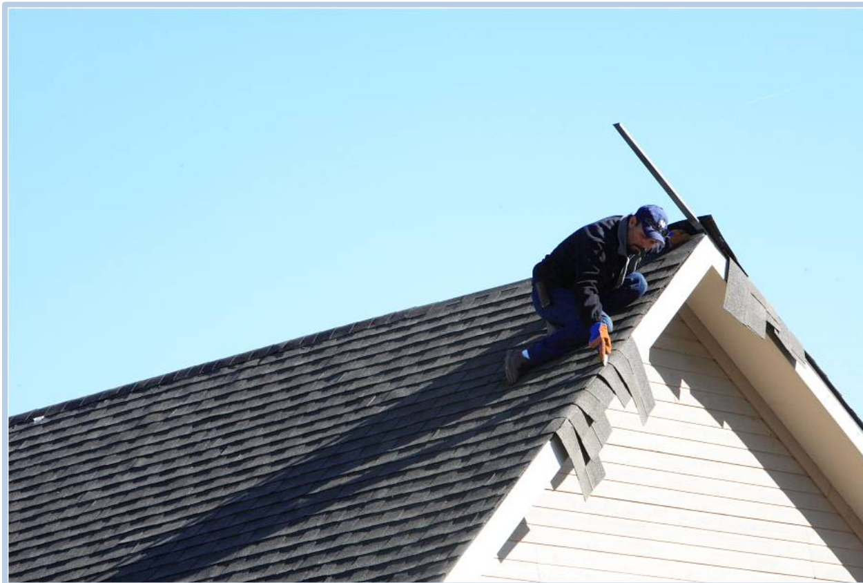
Roofer not using fall protection working on a steep-pitched roof.
