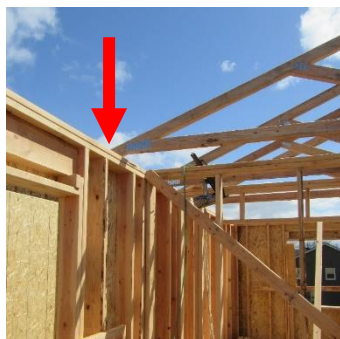
Interior view of house. The arrow points to where the framer was likely standing when he fell.
