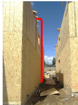
Location where framer fell.
