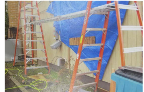
Extension plank on two ladders set up at the worksite with the plank staged at approximate height the carpenter fell.
