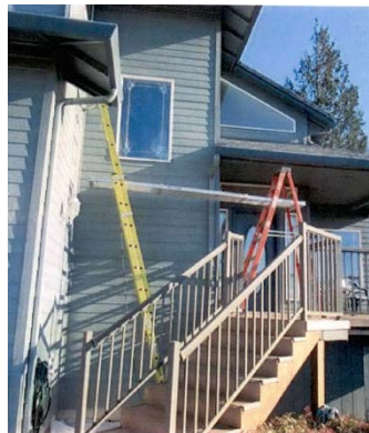
Picture of an extension plank supported incorrectly between two different ladders.
